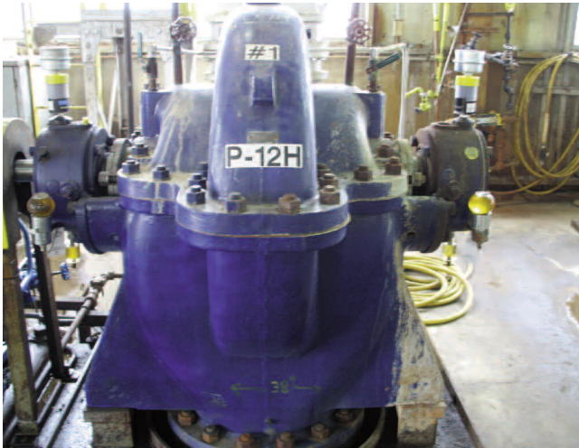
Figure 5. Between Bearings Pump with Composite Wear Rings Installed.
